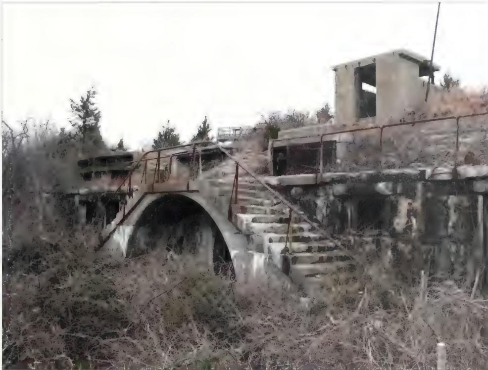
Figure 5.39. View looking northwest at Battery Peck. Today the area south of Battery Peck is filled with dense vegetation and is nearly impassable. Existing vegetation should be removed to resemble the open character present during the battery's years of operation and to improve access (Olmsted Center, January 2009).
